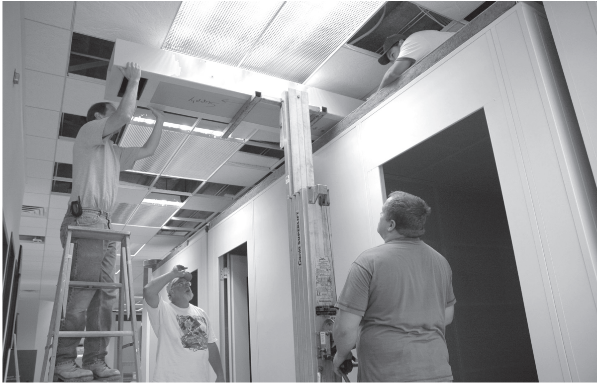
Team work — Project team members Joe Scanlon (lower left), Paul Lower (right) and Paul Reynoso (in ceiling) help Thomas Farrar of Acoustic Systems install noise-reducing air ducts in the ceiling of the new WRVO studios in Penfield Library. The seven-man project team has become a “go-to” group in many phases of the more than $100 million in campus renovation projects.
