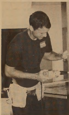
Campus carpenter Michael DeBonis prepares new walls for the relocation of Health Services to the Science Building.
